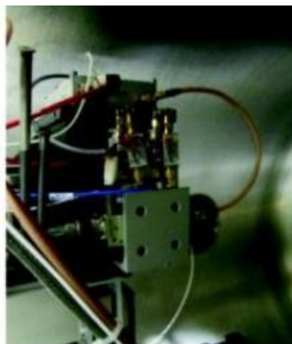
b) Support electronics (as ballast)
